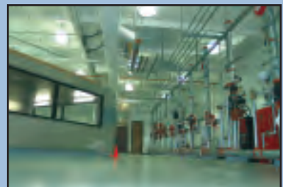
Valve lab and fire sprinkler test cell
